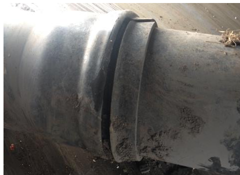
Figure 2: Force main pipe break.
