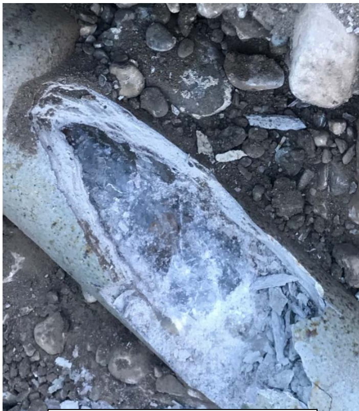
Frozen Sewer Main on Lawrence Street.
