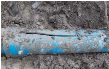
Water Break at Chief Mountain Ave.
