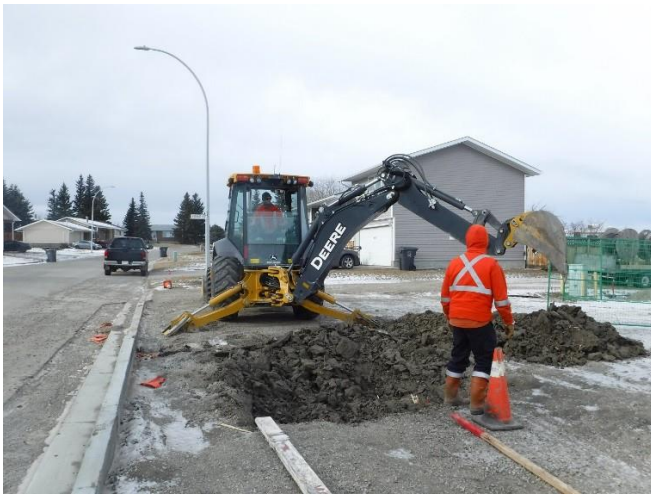
Underground Power Installation
