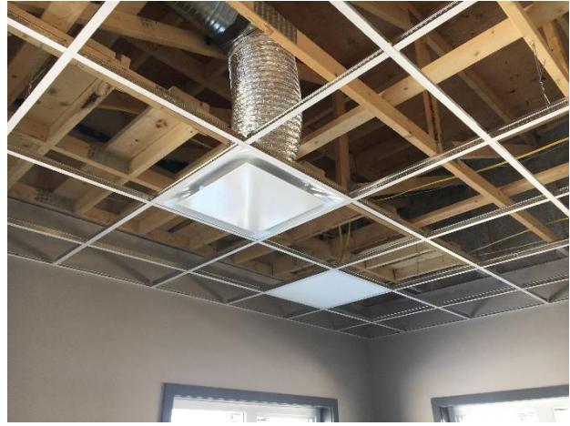
T-Bar Ceiling with H-Vac and Lighting
